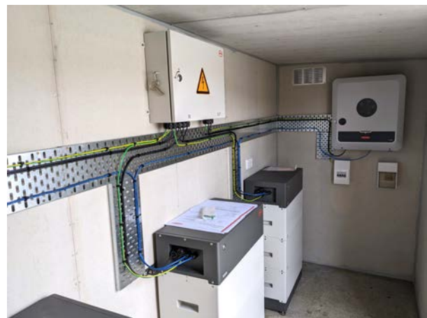
The battery stacks and control box in the enclosure adjoining the community centre built by the Men's Shed crew
